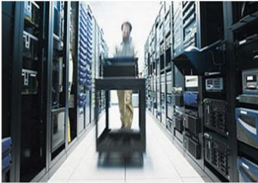
Uninterrupted Power Supply
